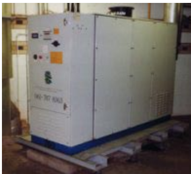
Small-scale CHP system
