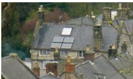
Poorly sited PV panels.
